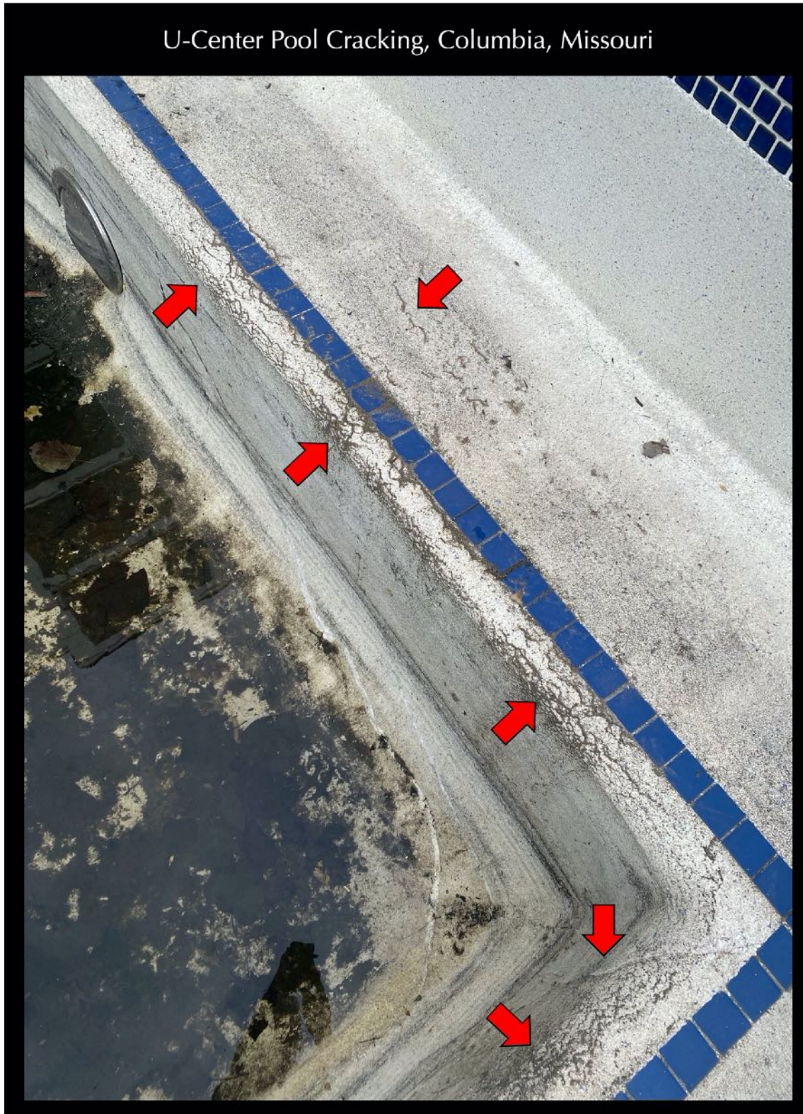
Figure 5: Both long, continuous, and short discontinuous cracks marked by red arrows. Many cracks have traversed through the steps and walls to the floor.
