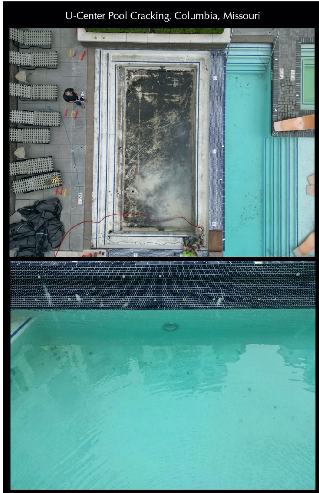
Figure 2: Field photos of pool from where four composite cores of pool plaster and shotcrete were retrieved.
