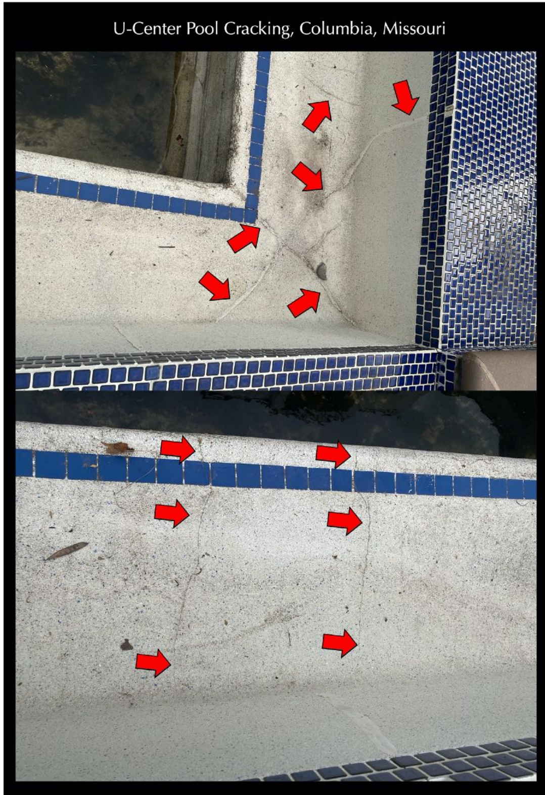
Figure 6: X-shaped intersecting cracks at the corners (top) along with long, vertical cracks on the plaster walls (bottom) marked by red arrows.
