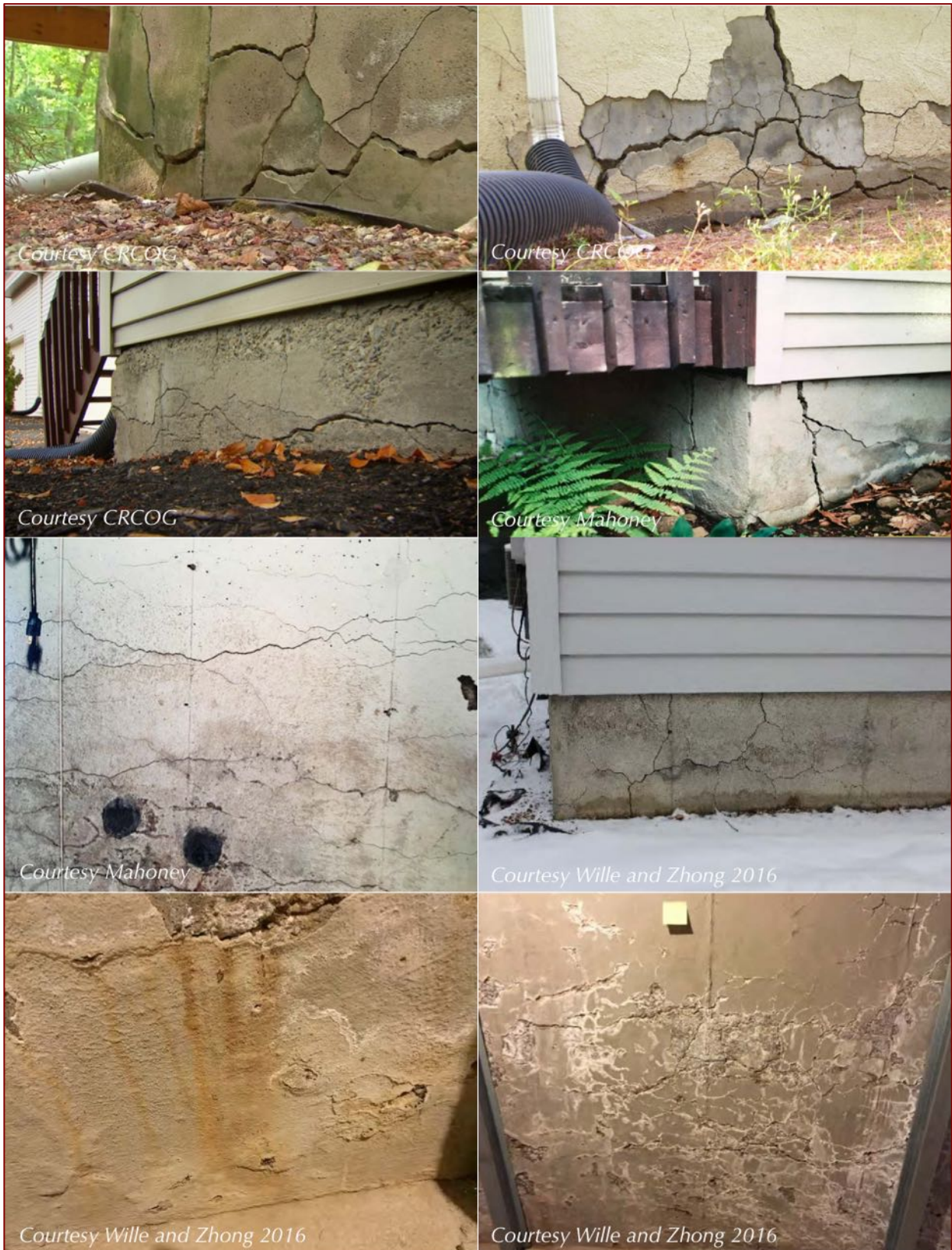
Figure 61: Cracking of concrete foundations in Connecticut due to oxidation of pyrrhotite bearing aggregates in concrete. Notice wide cracks in the top row as well as a network of numerous fine cracks in the wall in the bottom right row all from pyrrhotite oxidation and associated expansion of concrete.
