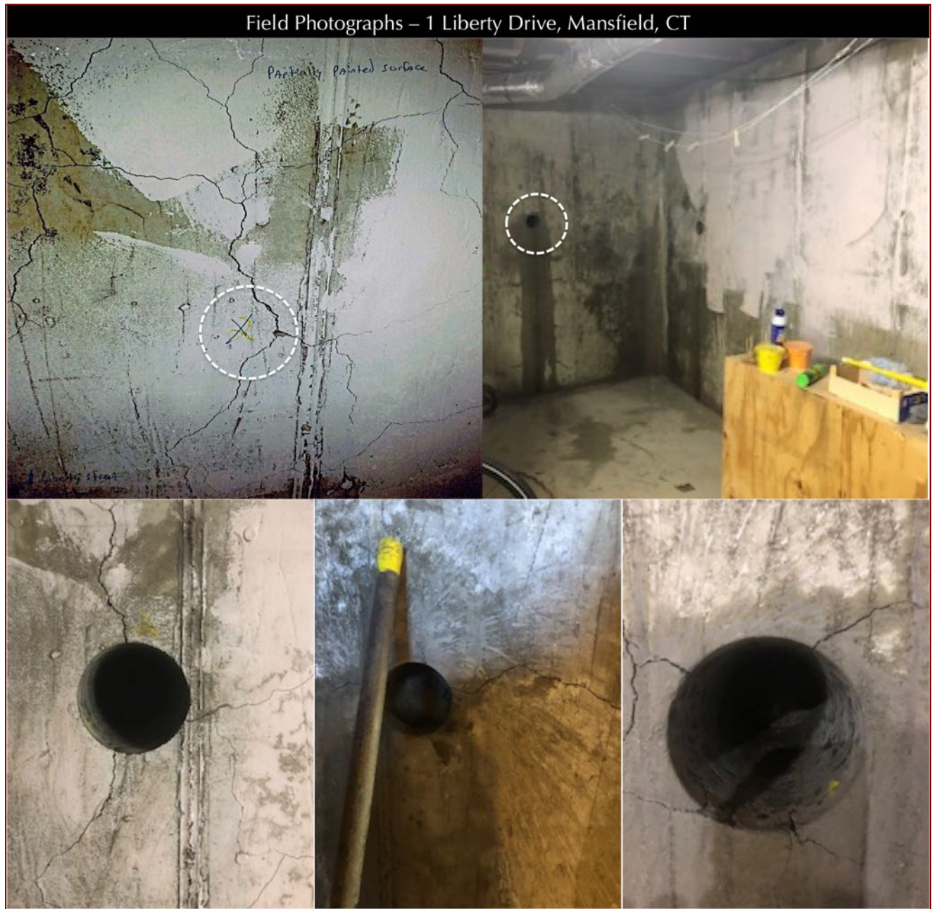
Figure 1: Field photographs of concrete foundation at 1 Liberty Drive showing extensive cracking of the foundation wall, overall closed polygonal-shaped pattern of many visible cracks, and location of the core for the present study retrieved from over visible radial cracks. Notice extension of the crack across the wall thickness at the core hole in the bottom photos, which is more clearly shown in the photos of the core when received in the laboratory.
