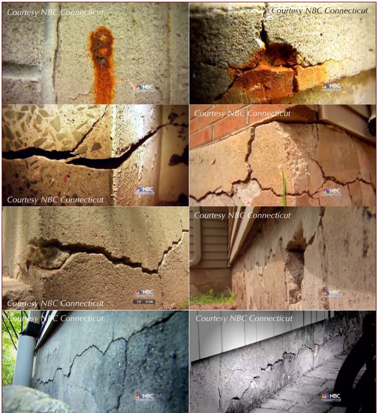
Figure 62: Cracking of concrete foundations in Connecticut due to oxidation of pyrrhotite bearing aggregates in concrete. Notice dark reddish-brown rust staining on the wall and associated cracking in the top row from pyrrhotite oxidation and formation of ferric oxy-hydroxide oxidation products (goethite, limonite, ferrihydrite rust minerals). Notice wide cracks in the 2 nd through 4 th rows from pyrrhotite oxidation and associated expansion of concrete.
