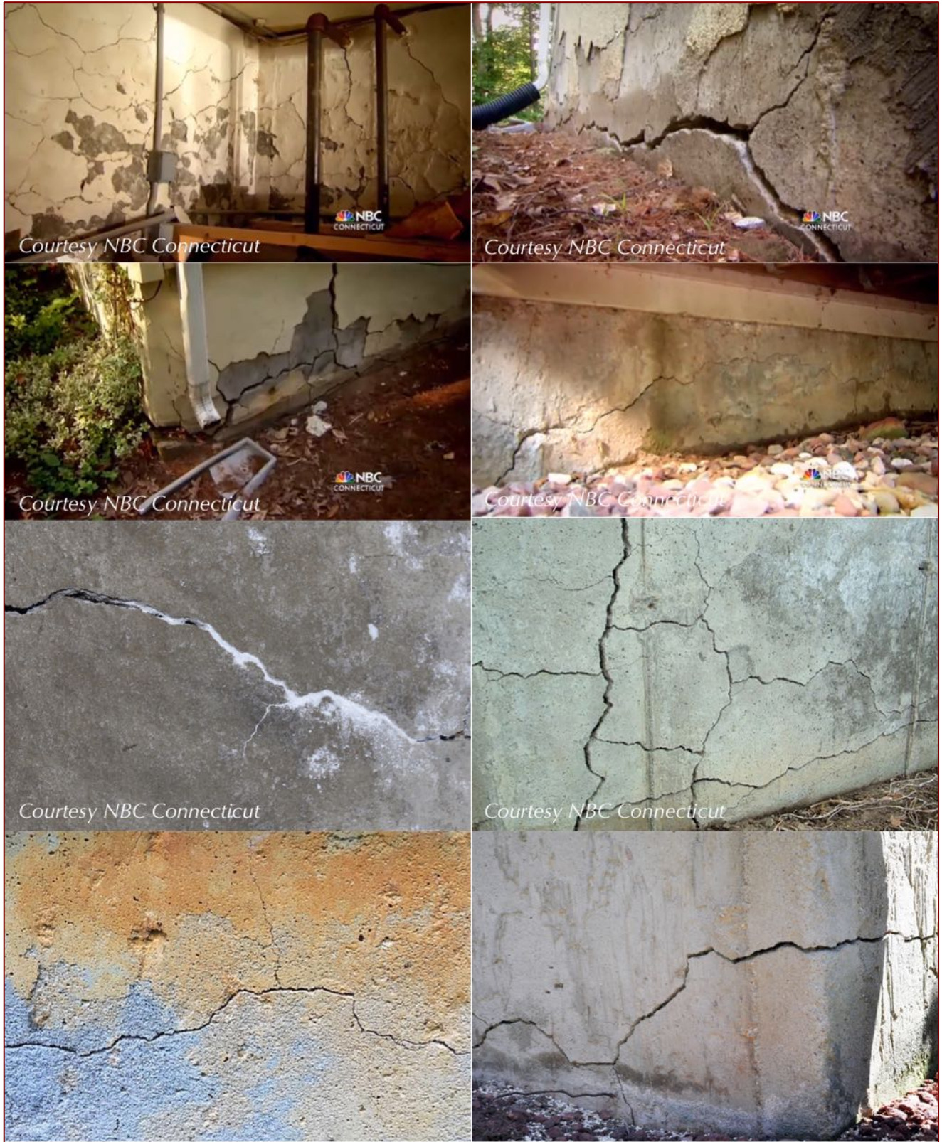
Figure 63: Cracking of concrete foundation in Connecticut due to oxidation of pyrrhotite bearing aggregates in concrete. Notice wide cracks in the foundation walls, extensive cracking of walls in the top left photo all reportedly from pyrrhotite oxidation and associated expansion of concrete.
