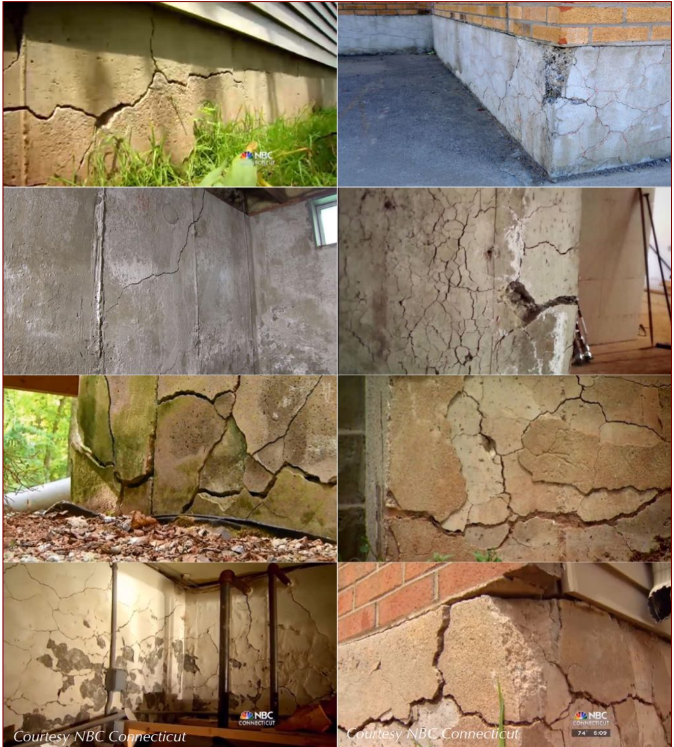
Figure 64: Cracking of concrete foundation in Connecticut due to oxidation of pyrrhotite bearing aggregates in concrete. Notice extensive cracking of foundation in all photos reportedly from pyrrhotite oxidation and associated expansion of concrete.
