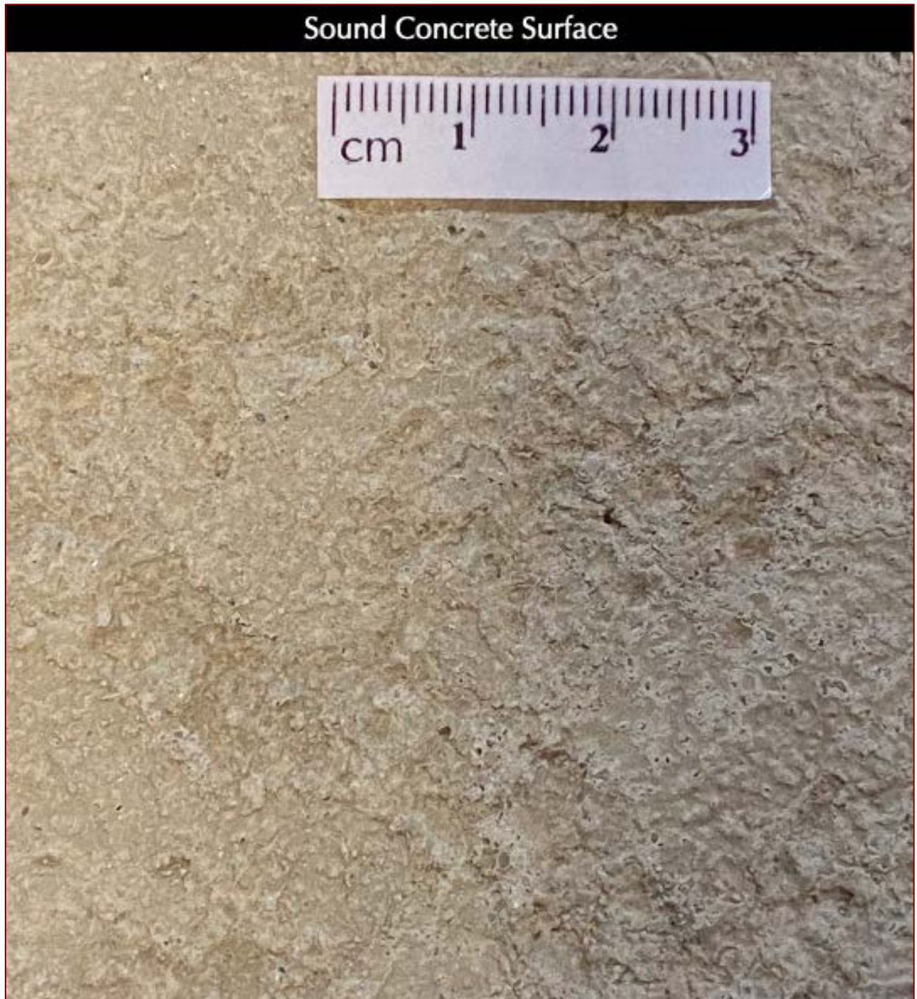
Figure 2: Enlarged view of the top exposed surface of the core collected from a sound location. The surface shows no loss of the original finished surface as seen in the core from the scaled area hence no exposure of near-surface coarse and fine aggregate particles. The original finished surface shows a light shiny appearance under reflected light indicating a possible application of a cure-seal compound after finishing.
