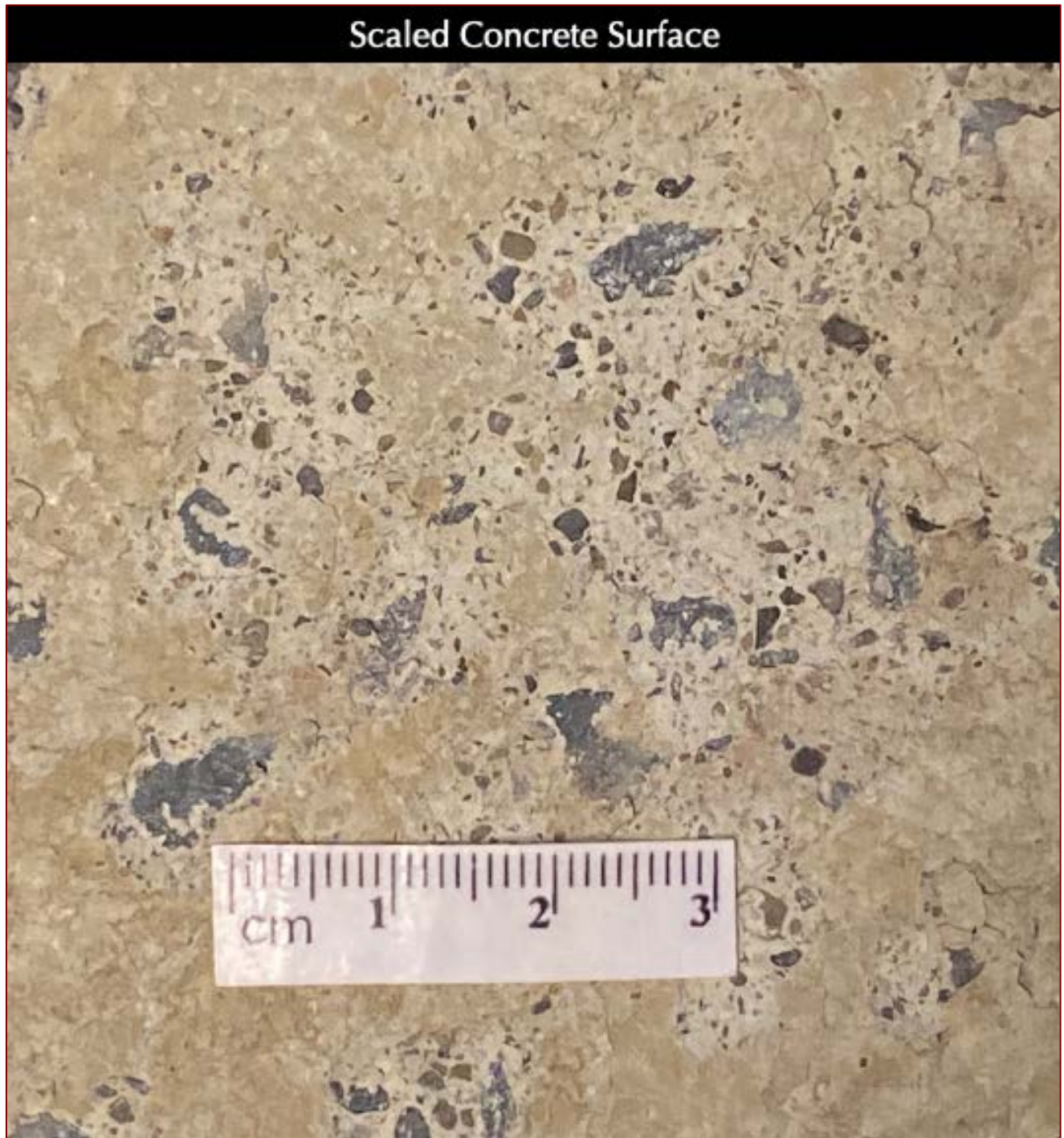
Figure 1: Enlarged view of the top exposed surface of the core collected from a scaled location. The surface shows losses of the original finished surface at isolated locations and exposures of near-surface coarse and fine aggregate particles from such losses. Remains of the original finished surface are still seen at some places, which show a light shiny appearance under reflected light indicating a possible application of a cure-seal compound after finishing.
